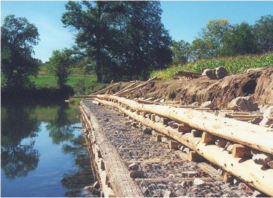
Nearly completed cribbing project. Note a buffer zone kept between the corn and the top of the bank.
